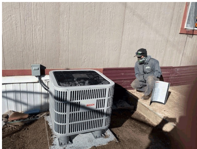
Air Supplied Heat Pump being inspected by NWCCOG Energy Program Team Member
