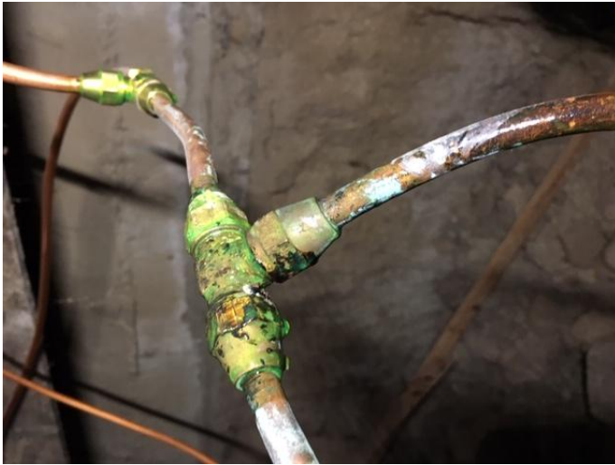
Leaking, corroded gas line.
