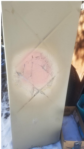
The cracking in the back of this furnace was close to causing a fire in the mobile home which could have been disastrous. See next photo.
