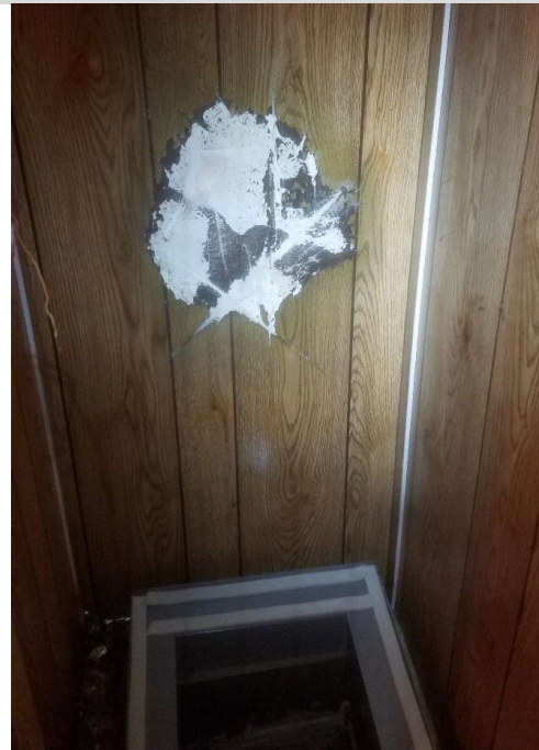
It's easy to see where the crack in the back of the previous photo's furnace, lined up to this wall in the mobile home -- it had very nearly burned through - and our auditor found the problem just in time.
