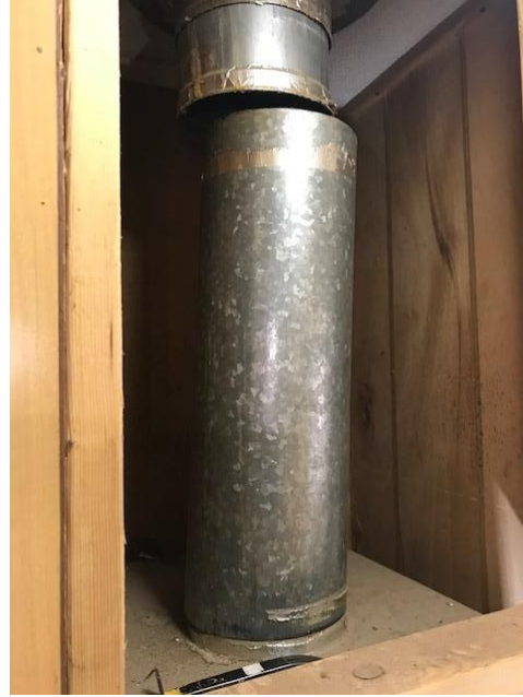
This flue not aligning at the top allowed dangerous fumes into the house and likely resulted in flu-like symptoms for the occupant until it was properly repaired.
