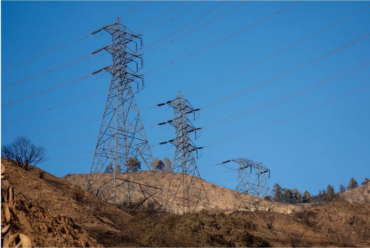
Southern California Edison transmission towers in Eaton Canyon that are under investigation as the possible point of ignition of the Eaton Fire. Photographer: Kyle Grillot/Bloomberg
